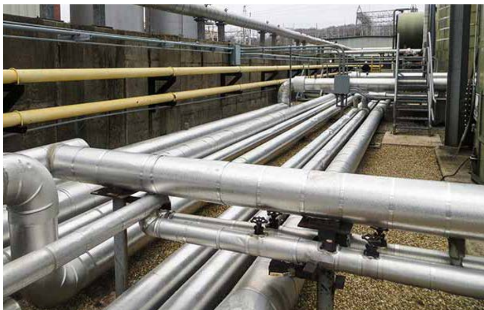
Image 1. Long suction piping from horizontal tank in background. (Images courtesy Kristo Naude)
